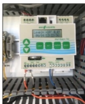
Control unit shown DIN-rail mounted in electrical enclosure
