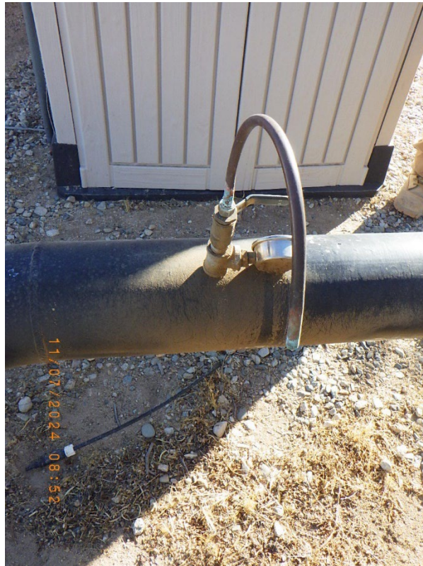
Figure 03: Sample tap after the check valve
