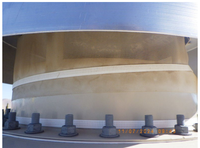
Figure 13: Vent on East tank
