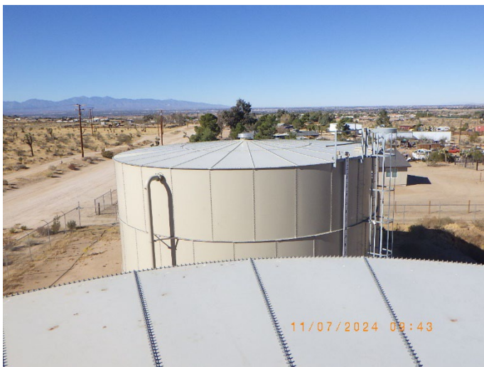
Figure 12: Top of both East & West tanks
