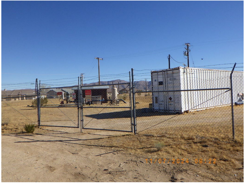
Figure 10: Fence around both wells and storage
