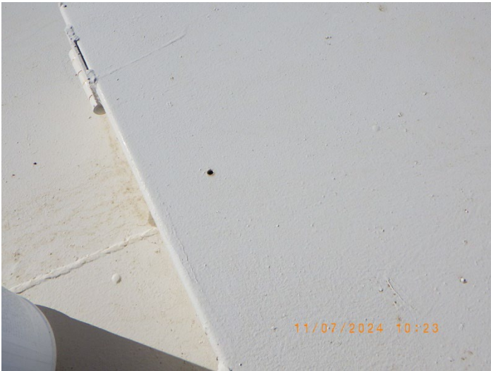
Figure 16: Tank hatch has a small hole
