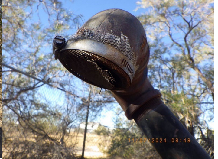
Figure 02: Current mesh is ripped. Install a new screen mesh.
