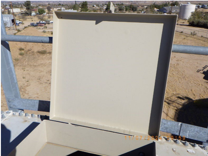
Figure 14: Both tank hatches missing gasket
