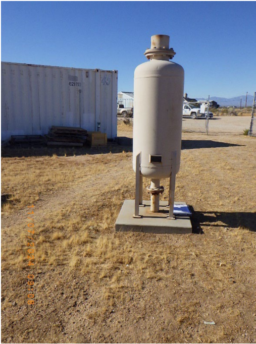
Figure 09: Bladder Surge container Arrestor Tank
